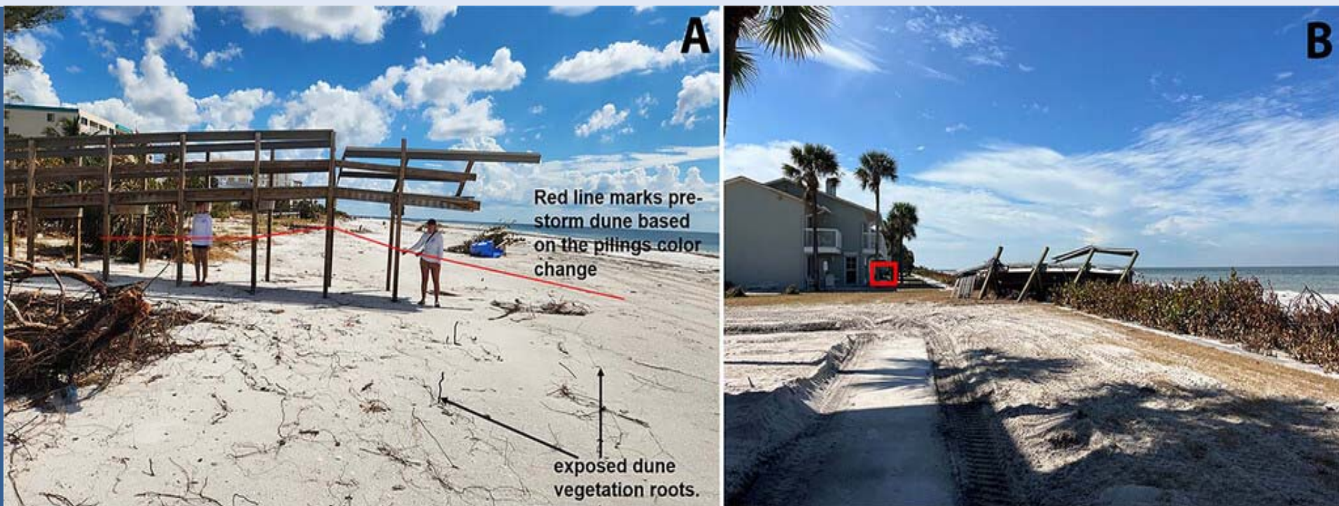
Figure 6. Damage to dune overwalk by Hurricane Helene. (A) Severe beach and dune erosion at an overwalk, the part with the stairs could not be found in the nearby area; (B) part of a dune overwalk was washed over the seawall and crashed into a beach front building (red box).
